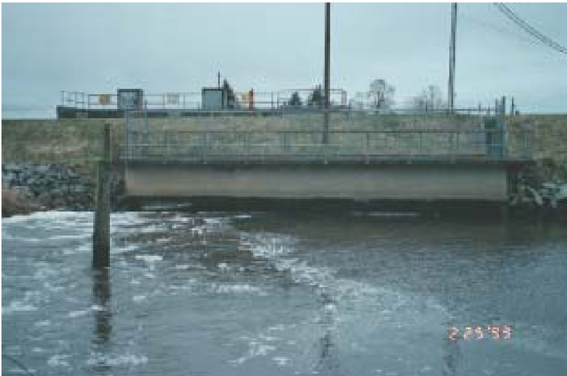
Photo 4: Katie Slough station: pump and flood box outfall.
