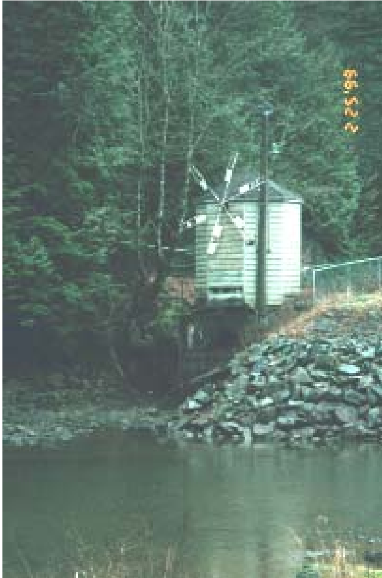
Photo 10: Miami Creek pumping station: old flood boxes under station. Also note the aged screen in front of the sump.
