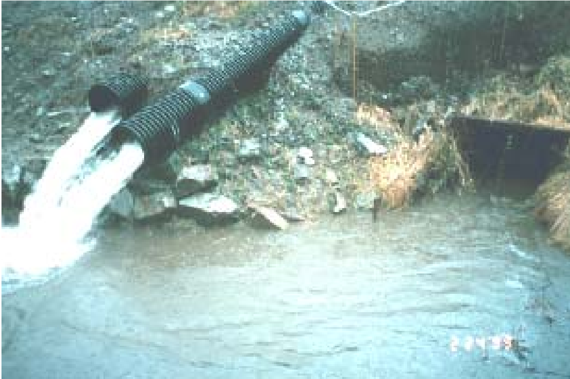
Photo 23: Lane Creek station: pump (L) and flood box (R) outfalls.
