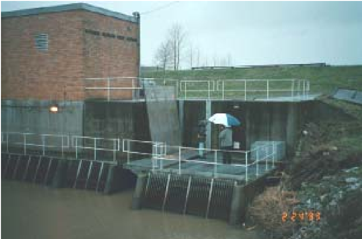
Photo 5: Matsqui Slough station: fish pump and screen located in right forebay.
