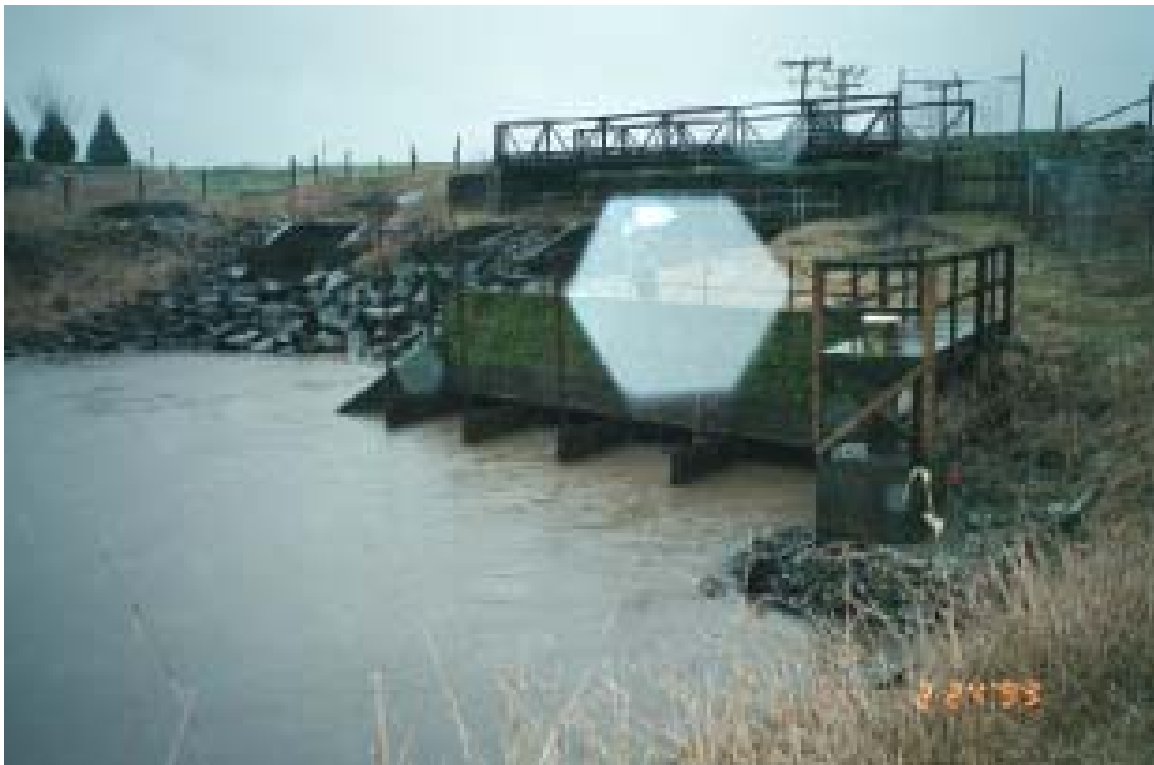
Photo 6: Matsqui Slough station: flood box outfall (R), pump outfall (L).
