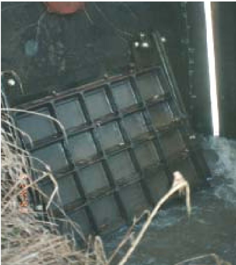
Photo 20: Silverdale station (Chester Creek): new top mounted steel flap gate on flood box outfall.
