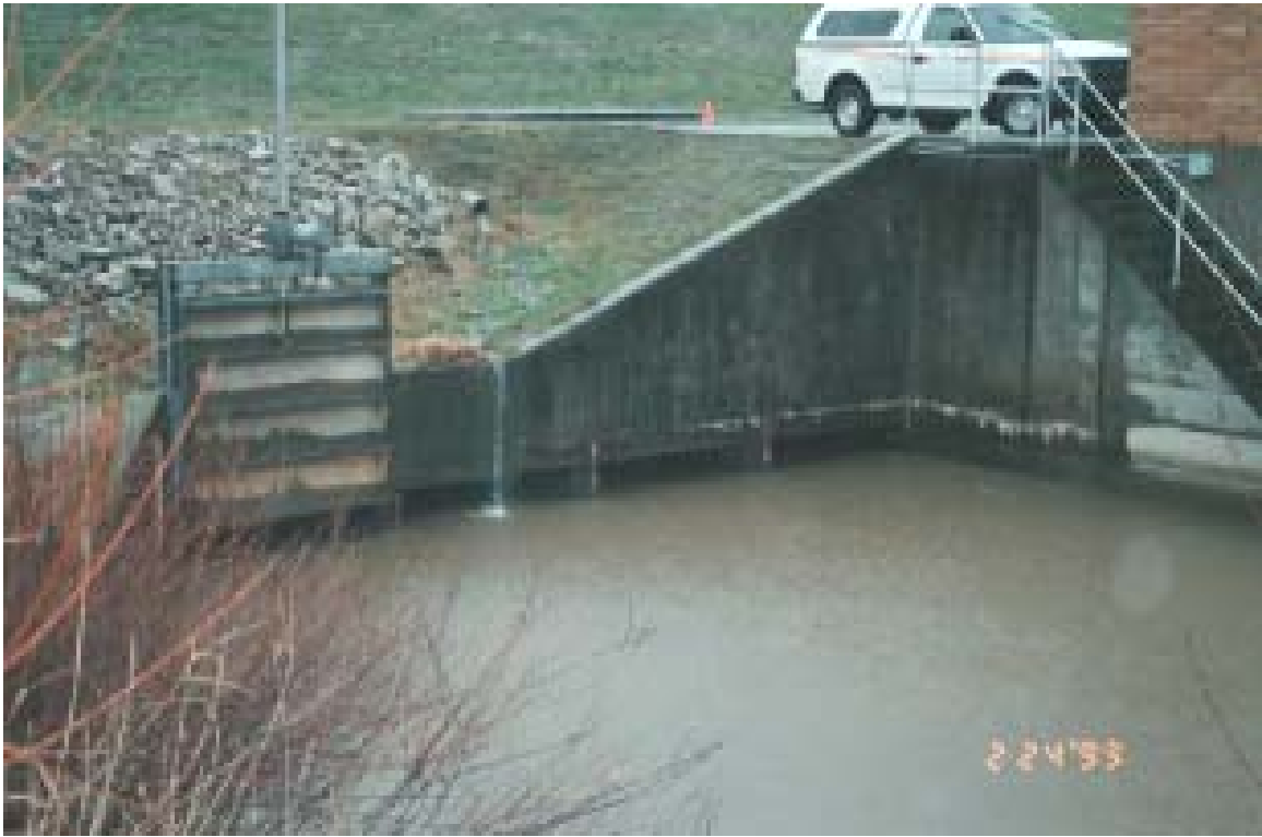
Photo 7: Matsqui Slough station: entrance to flood boxes. Note hydraulic gate and slots for stop logs.
