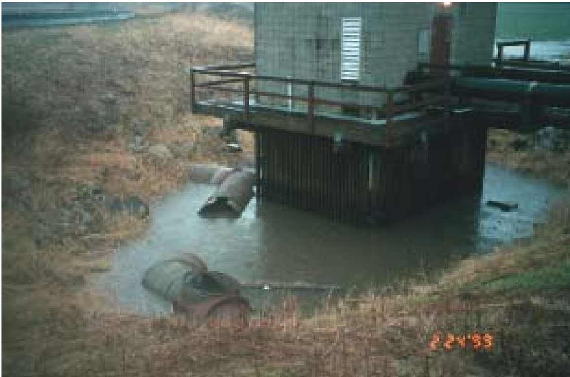
Photo 21: Lane Creek station: Lane creek enters through culvert in center of pic.
