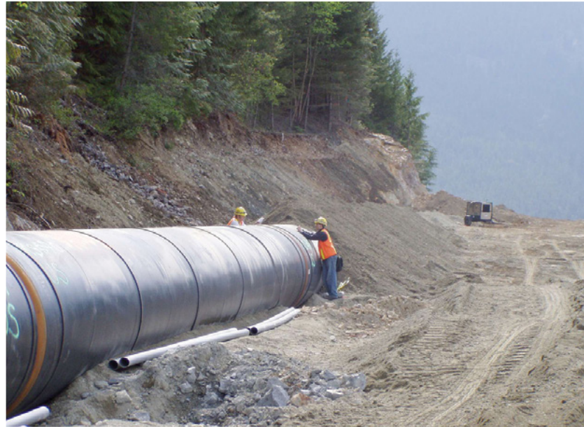
Penstock being laid for the 2003 Rutherford Creek river diversion project near Pemberton, BC
