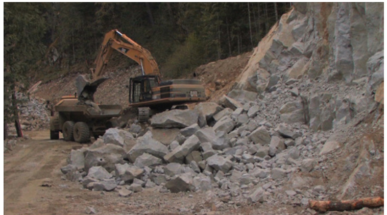
Road building and blasting for the Tipella Creek river diversion near Harrison Lake
